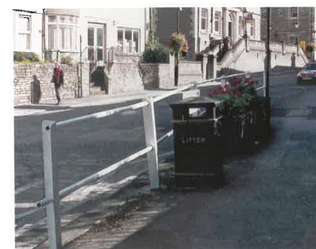
Areas of raised pavement are poorly maintained with railings and surfaces disrupted and not consistent. Project 36a to 37b
