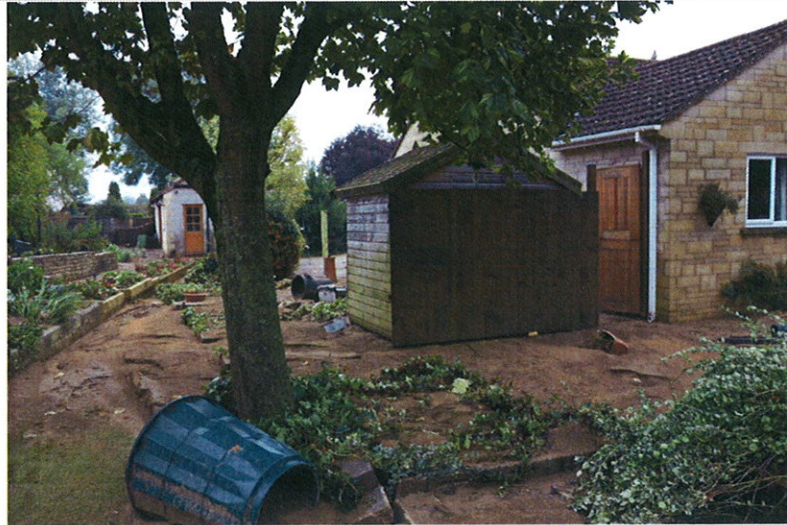
Figure 4: The collapsed garden wall between [REDACTED] (on the right) and [REDACTED]. The wall stood just to the left of the wooden shed.
